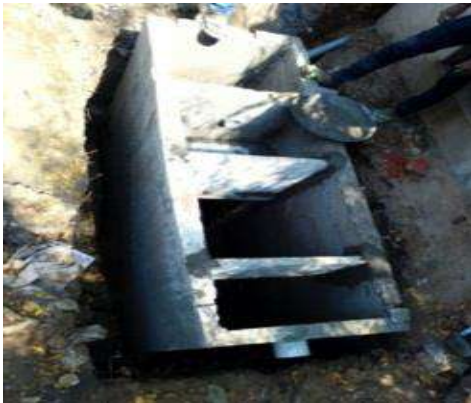
Bargarh Sabar Sahi Septic Tank
