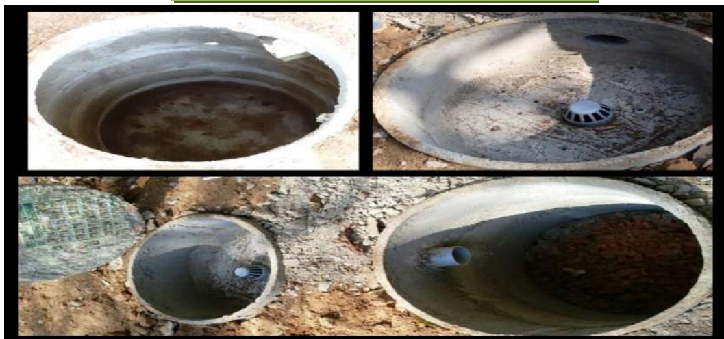
Anganwadi Ring Septic Tank
